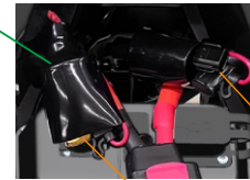
Low voltage fuse box (black)
